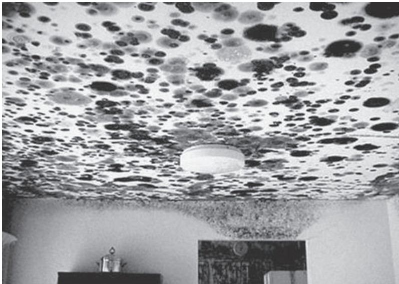
FIGURE 6–7 Excessive mold growth on the ceiling of a water damaged residence. Photo courtesy of the Centers for Disease Control and Prevention. Available at: http://www.cdc.gov/nceh/publications/books/housing/Graphics/chapter_05/Figure5.01.jpg .
