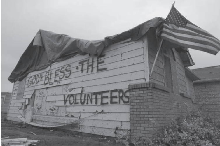
FIGURE 1-6 Windsor, Colorado, May 26, 2008—The message written on the side of this home is a result of volunteers who came to Windsor to help residents recover from the recent tornado. Photo by Michael Rieger/FEMA.
