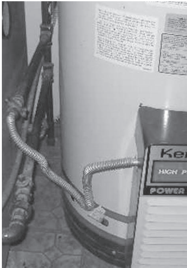
FIGURE 5-7 Flexible gas line connection on a water heater.
