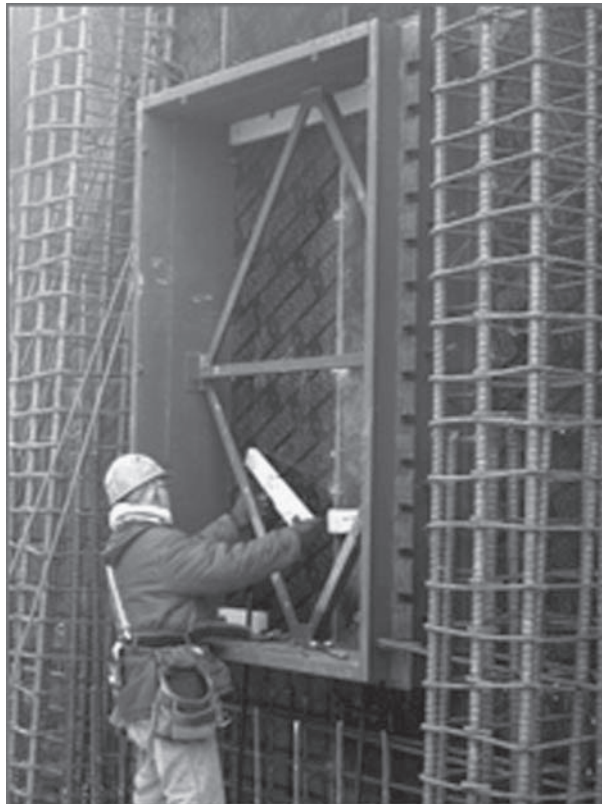
FIGURE 3–6 A contractor installs a blast-resistant window frame in the outer facade of the Pentagon's E-ring.
