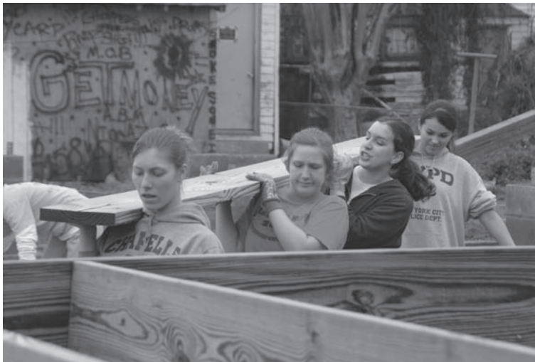
FIGURE 1-5 New Orleans, LA, January 21, 2006—Volunteers from AmeriCorps carry a floor joist at a Habitat for Humanity home site in New Orleans. The organizations have teamed up to provide housing for Hurricane Katrina victims. Volunteer agencies are important FEMA partners who provide needed service to victims. Photo by Marvin Nauman/FEMA.
