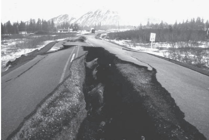
FIGURE 5-5 Alaska Earthquake, March 27, 1964. This highway embankment fissured and spread as a result of liquefaction. The road was built on thick deposits of alluvium and tidal estuary mud. Image courtesy of U.S. Geological Survey. /htmllib/batch07/batch07j/batch07z/batch07/aeq00065.jpg .
