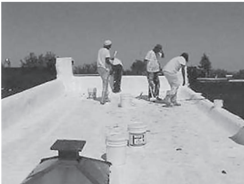
FIGURE 7-8 Workers apply cool roof coating on a row house in Baltimore, MD. Source: EPA. http://www.epa.gov/hiri/images/Baltimore.jpg .
