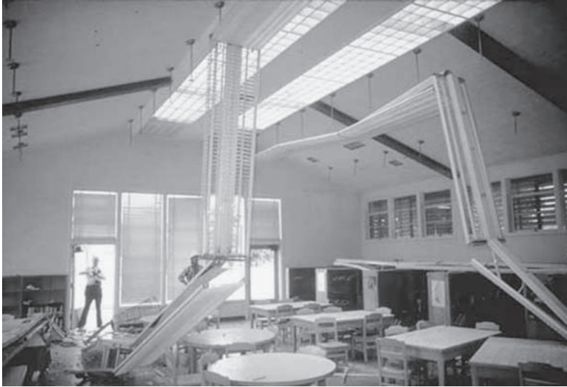
FIGURE 5-8 A classroom without braced light fixtures damaged by the 2001 Nisqually earthquake in the Puget Sound region of Washington. Photo courtesy of U.S. Geological Survey.
