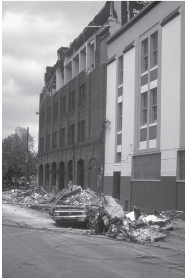
FIGURE 5–9 Loma Prieta, California, Earthquake, October 17, 1989. San Francisco. Cars crushed by a collapsed brick facade near 5th and Townsend. Five people were killed at this locality while leaving work. Source: U.S. Geological Survey Open-File Report 90-547. http://libraryphoto.cr.usgs.gov/html/lib/btch136/btch136j/btch136z/btch136/mce00001.jpg .
